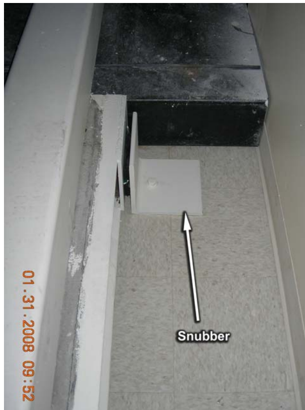
Figure 12: Snubber installed at end of inertia base to restrict lateral movement.
