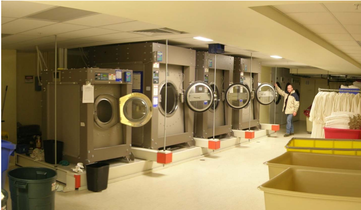
Figure 13: Washer/extractors on retrofitted inertia base.
