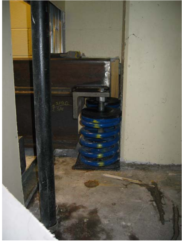
Figure 10: Spring isolator at rear of base at column.
