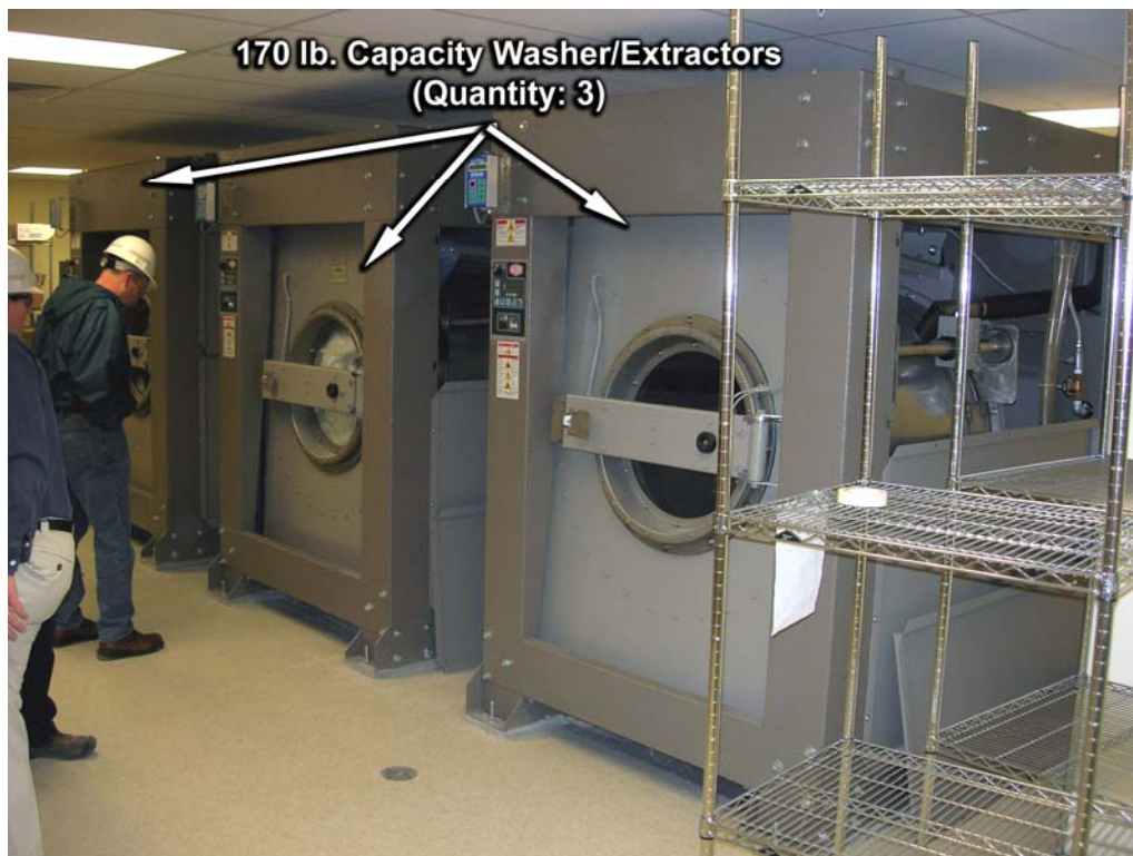
Figure 2: 170 lb. capacity washer/extractors as initially installed.
